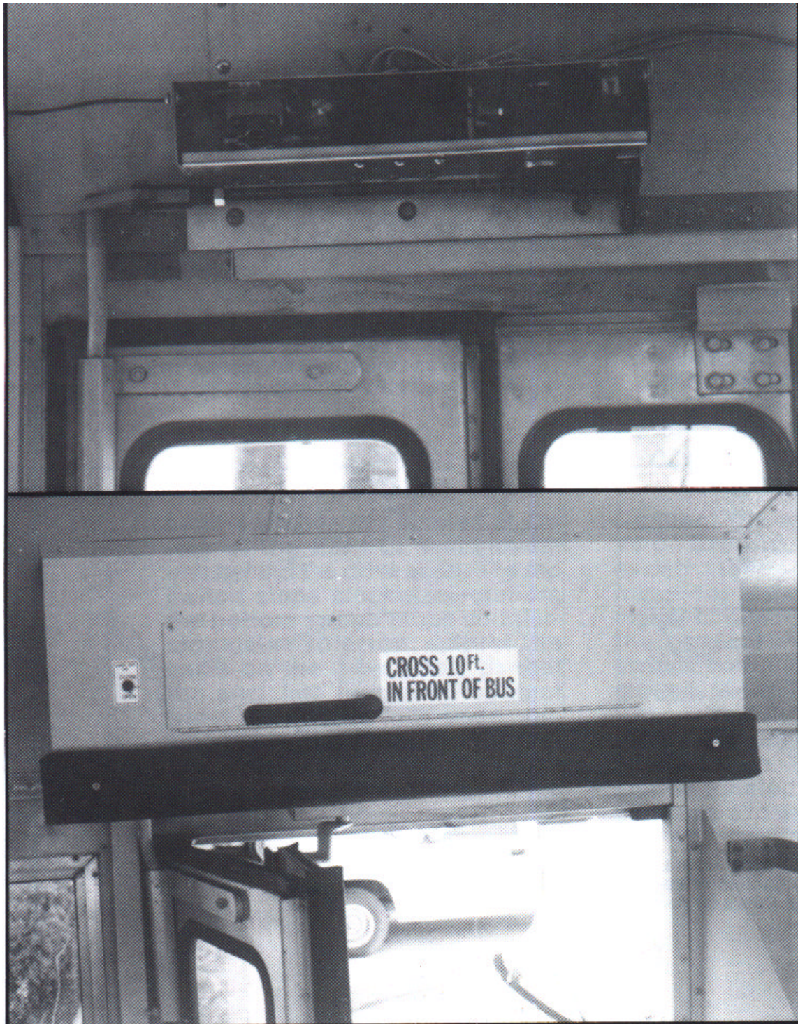
Figure 8 – Showing the Excell mechanism set to operate bi-fold doors on a Ward Patriot Bus. A standard retrofit mechanism was used to convert the door operation from air to electric, utilizing the existing drive brackets. Shown with cover on mechanism removed and doors closed, and with mechanism cover in place and doors open.
